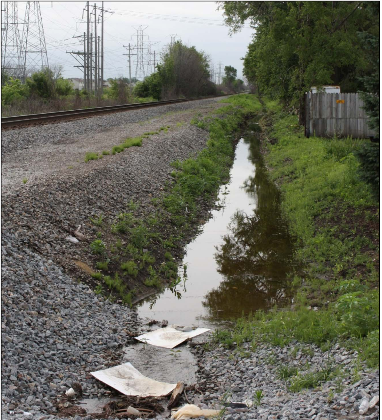
Culvert running at the base of the EJ&E tracks (spanning a distance of at least 600 feet.)
