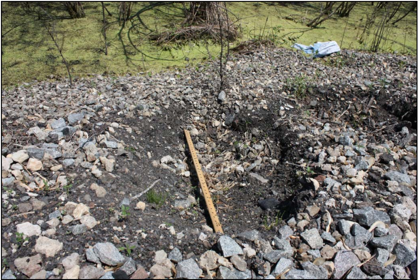
One of approximately 26 sinkholes near the EJ& E tracks (note green standing marshy waters at the top of the photo.) The sinkholes span a distance of approximately 300 feet. CN has filled them in with gravel at least five times since the spring of 2010.
